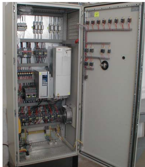
Fig.3. The AER 2x30 control cabinet..
