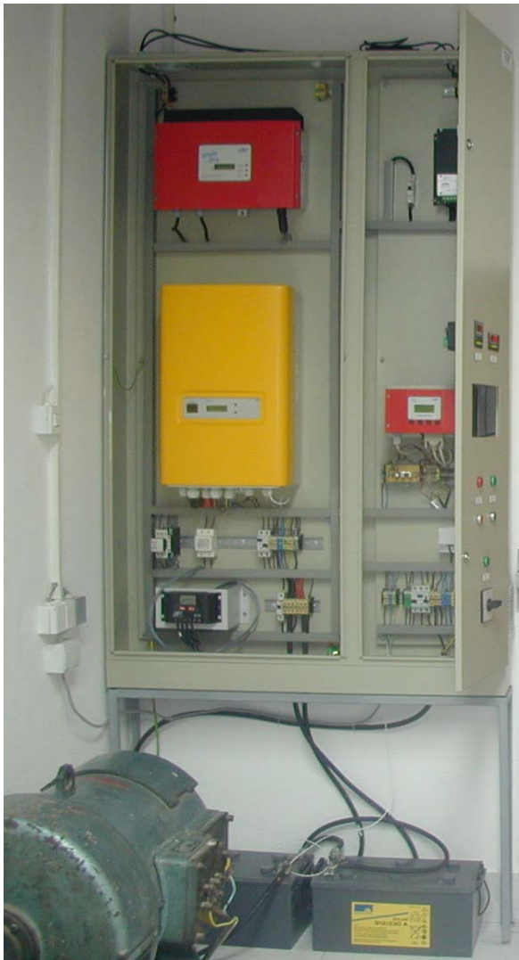
Fig. 8. Realized Hybrid system control board.
